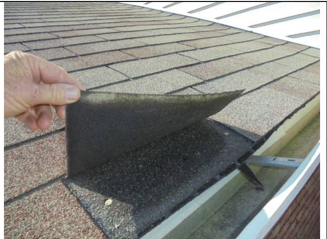
The leading edges of the starter row of shingles are not sealed at the eaves.
