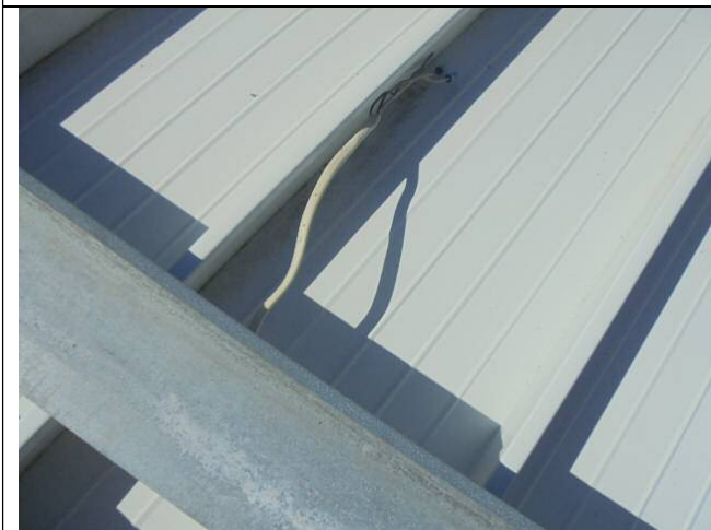
Abandoned wiring on top of the metal roof for the porch enclosure should be removed or appropriately terminated.
