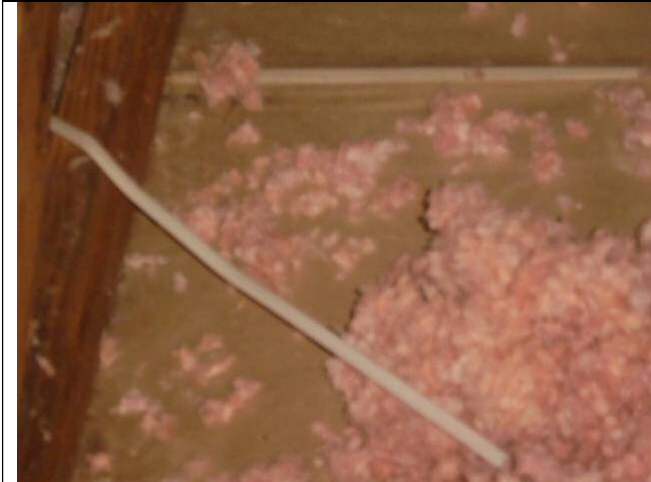
Insulation should be evened out. There are areas above the middle bedroom and hall that have no insulation.
