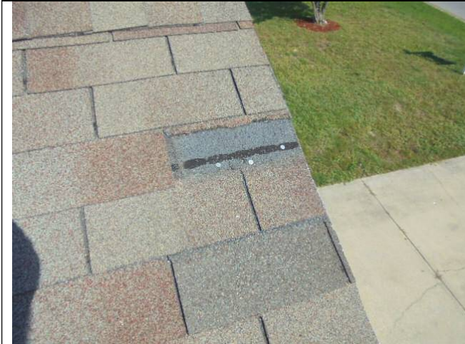
Missing shingles should be replaced as necessary.
