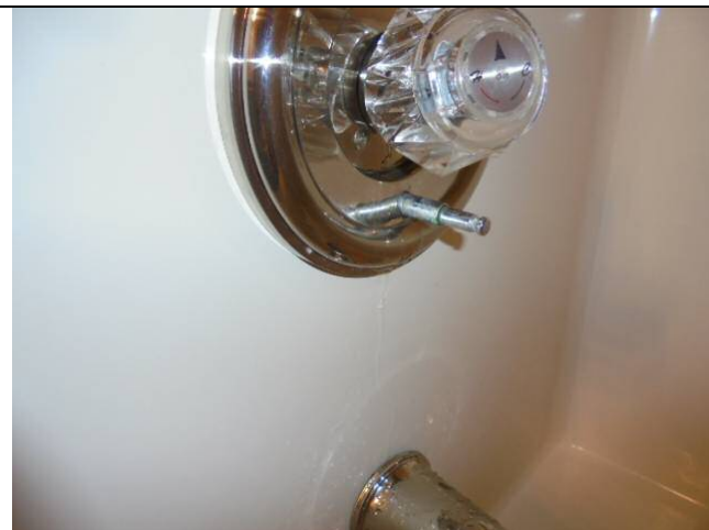
The bathroom tub and shower faucet(s) are leaking at the handle when the water is on.
