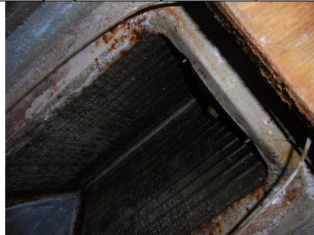
The interior coils were observed to be dirty and/or corroded. The cooling coils should be cleaned and/or leak checked as needed.
