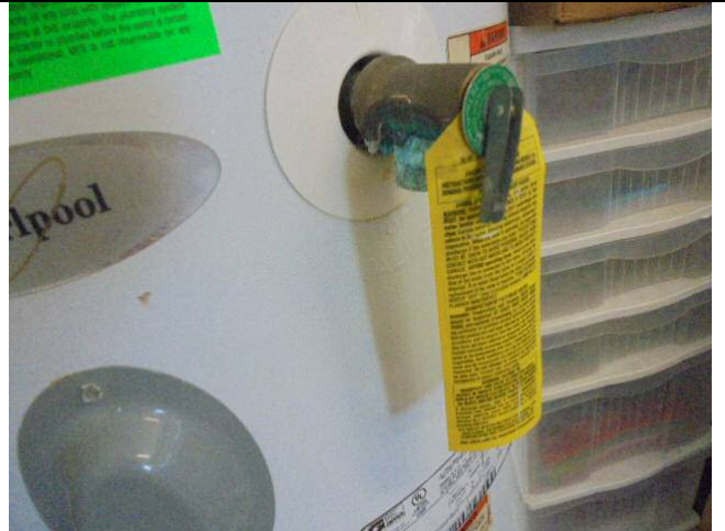
Discharge piping should be added to serve the Temperature and Pressure Relief (TPR) Valve for the water heater. It should terminate not less than 6 inches or more than 24 inches above the floor.
