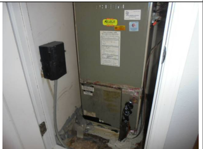
Many of the screws for the evaporator are missing and the interior components are in a state of disassembly/missing parts
